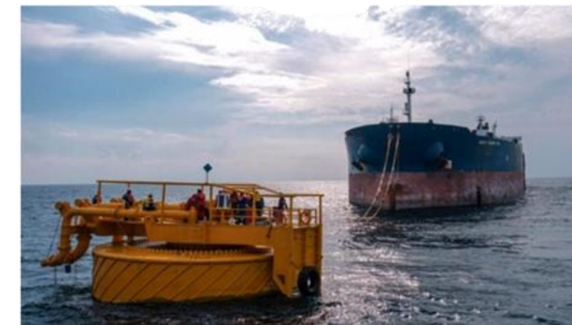
Single Point Mooring
